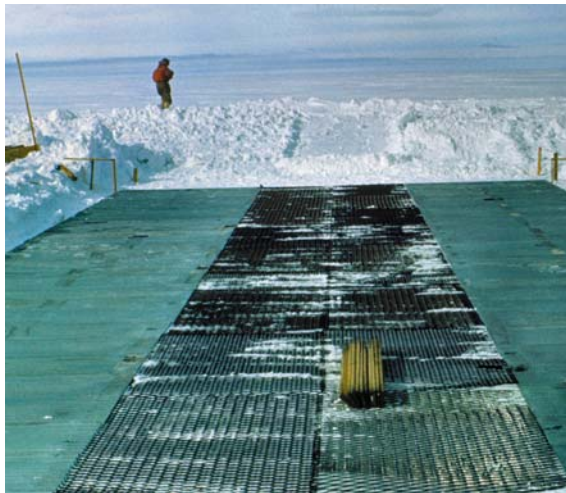
A bulldozer was used to level the site. The finished surface was tamped using screed boards. Galvanised corrugated sheets and galvanised mesh was placed on the level snow surface to form sub-foundations. (E.J. Chinn)
