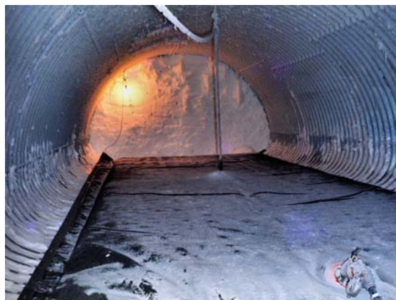
Picture to the right shows the Armco tube completed and housing the fuel oil flubber. This was the first time this type of bulk fuel storage had been used at Halley Bay (E.J. Chinn)
