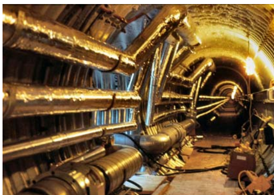
Picture to the left shows the Armco tunnel between ACB and ICB buildings and building services being installed January 1990 (A. Smith).
