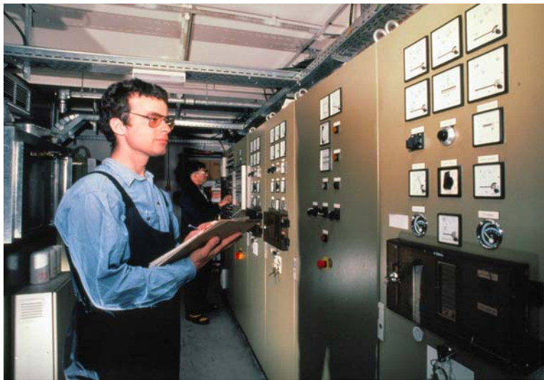
Picture to the left shows the generating and distribution panel. (P. Bucktrout)
