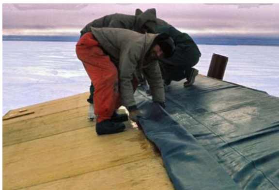
Picture to the left shows the Butyl sheeting being fixed to the roof panels using adhesive. This was very successful. (E.J. Chinn)
