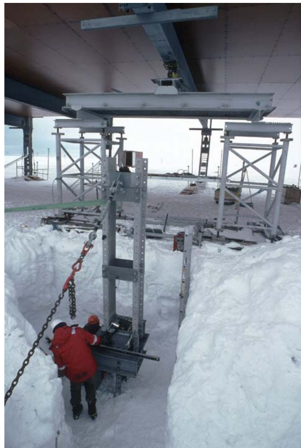
Picture to the right shows the two load-bearing towers temporarily supporting the main steel platform cross-beam and the column being exchanged 1993/94 season. (BAS)
