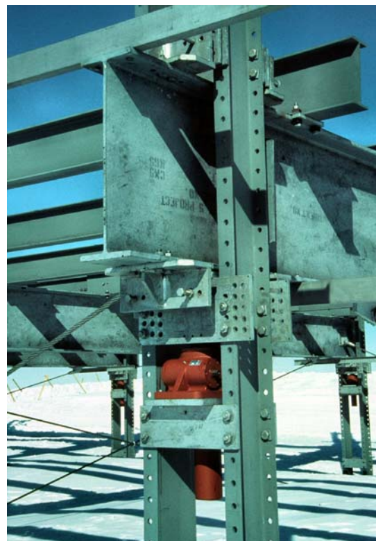
Picture to the left shows lifting steel cross beam into position to save manual jacking time. (A. Smith)
