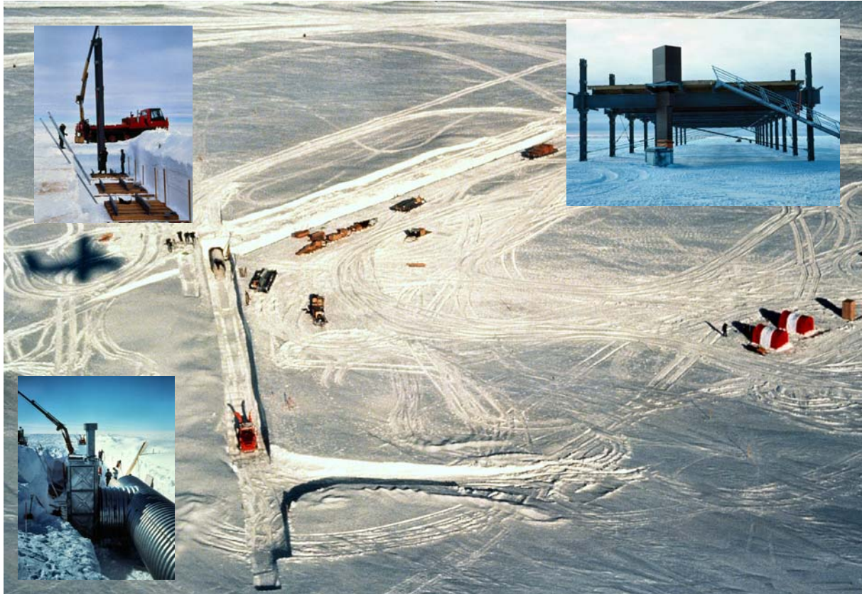
Commencement of excavations by rotary snow plough for the ACB platform foundations and sub-surface Armco tunnel between ACB and ICB platforms December 1988 (BAS).
